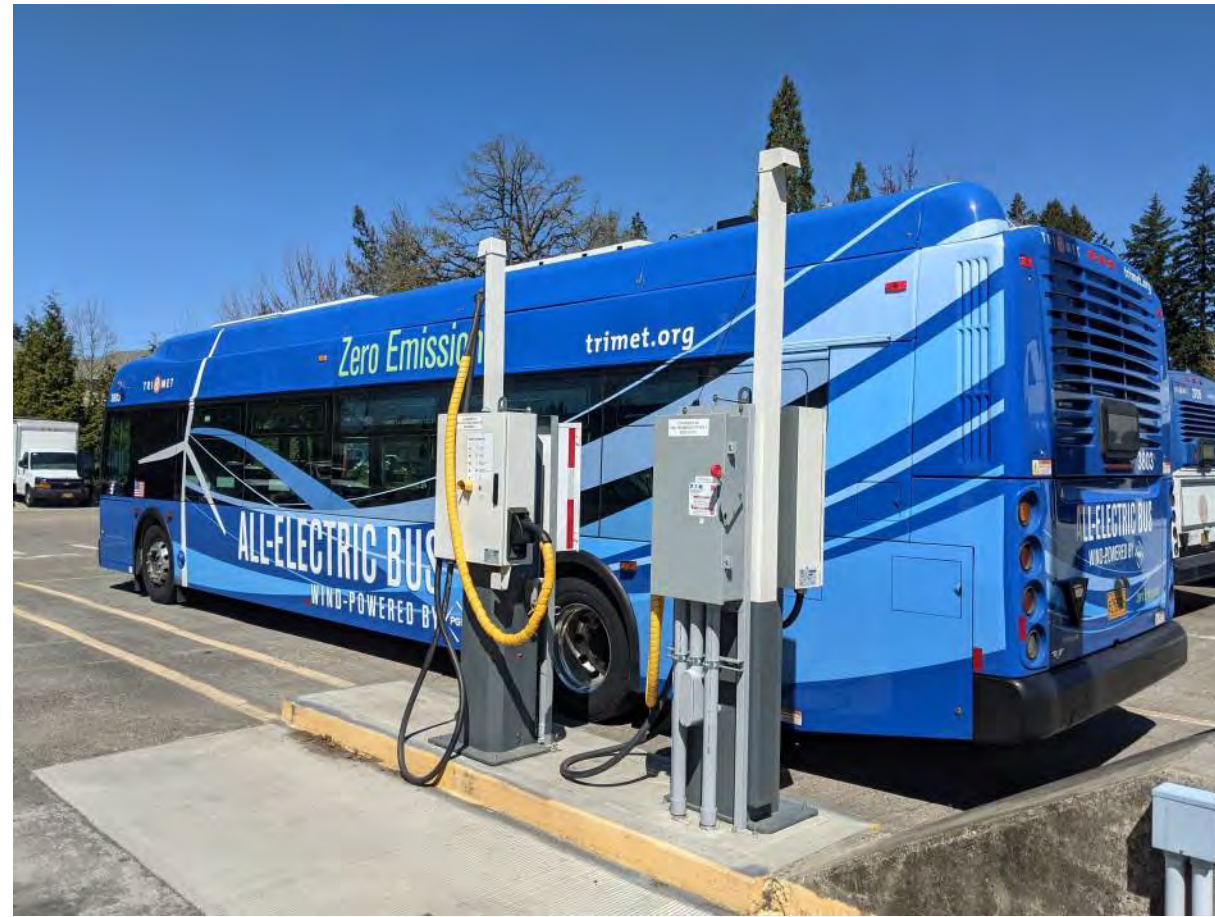
TRIMET MERLO - BATTERY ELECTRIC BUS (BEB) DISPENSERS
