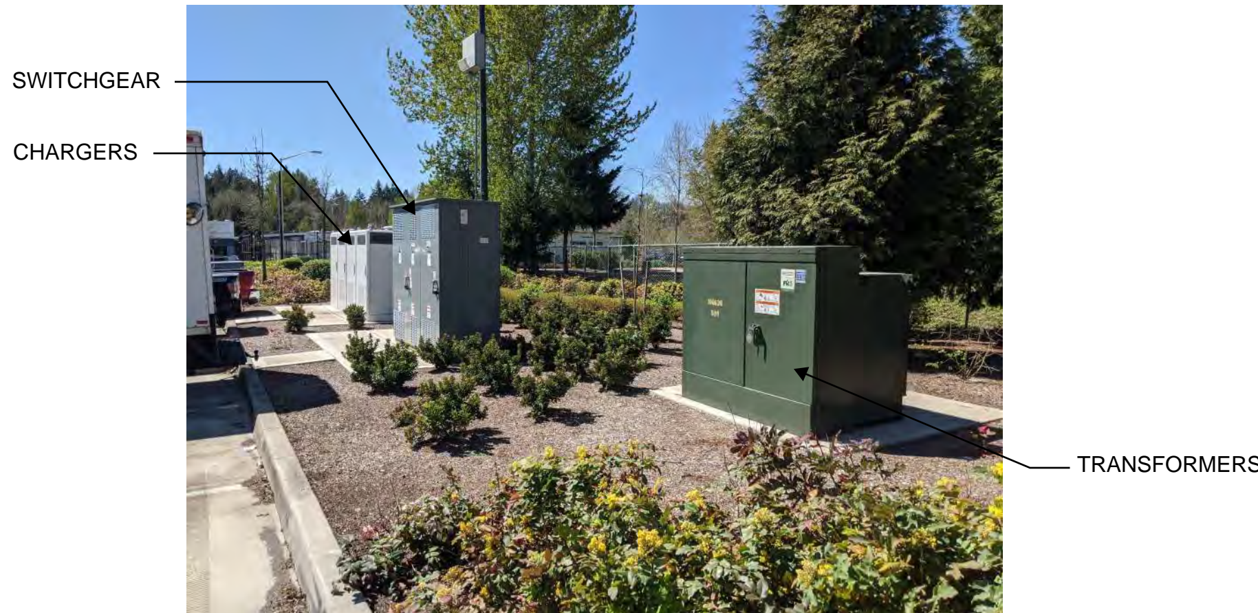
TRIMET MERLO - BEB INFRASTRUCTURE
