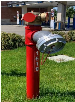
(Example of the FDC connection – pipe size to be determined by design)
